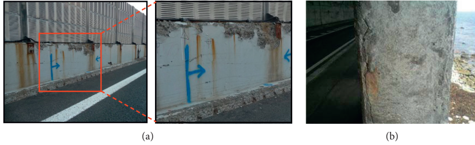
FIGURE 1: Frost damage in existing structures. (a) Damaged reinforced concrete (RC) wall barrier on the highway. (b) Damaged condition of RC pier of a rock shed.
