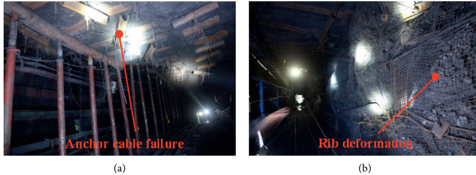
FIGURE 15: Deformation characteristics of the entry in San coal mine in Yangquan coal field. (a) Anchor cable failure. (b) Rib deformation.
