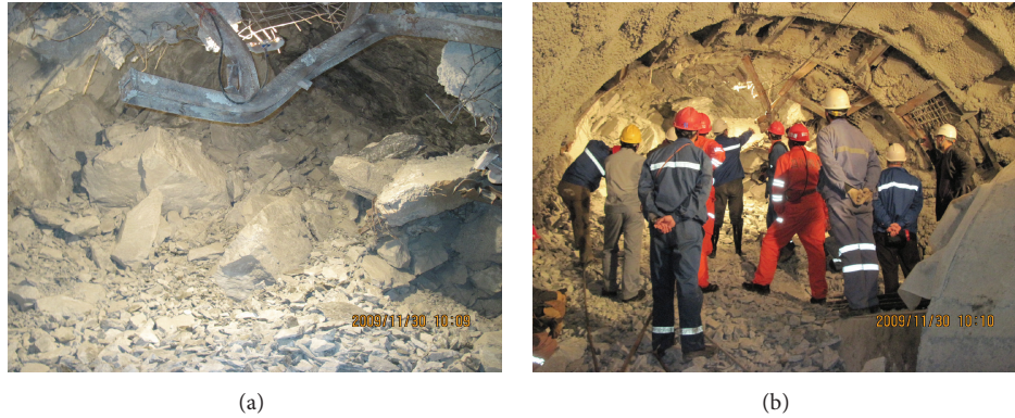
FIGURE 1: On-site photos showing strong rockburst failure in drainage tunnel at Jinping II Hydropower Station, Sichuan, China (November 28, 2009). (a) The support systems were seriously damaged and a large area of rocks burst and collapsed. (b) Experts investigated the accident scene after the strong rockburst.
