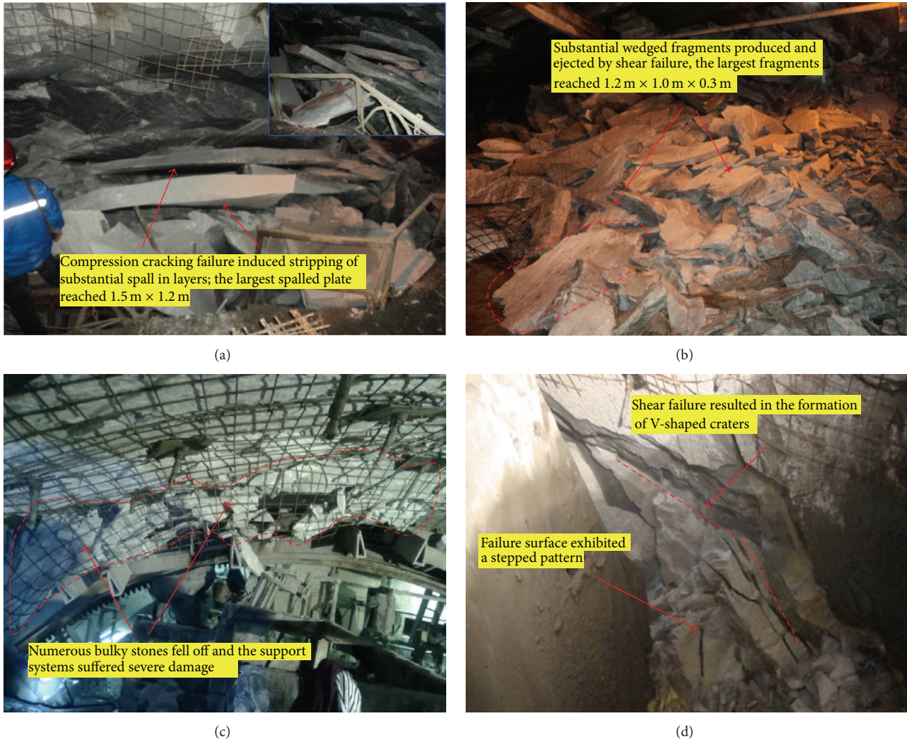
FIGURE 11: On-site photos showing the failure caused by rockburst. (a) Compression cracking failure induced stripping of substantial spall in layers. (b) Substantial wedged fragments produced by shear failure were ejected to a certain distance. (c) The anchoring-shotcreting and flexible support systems suffered severe damage. (d) Rockburst failure resulted in the formation of V-shaped craters.
