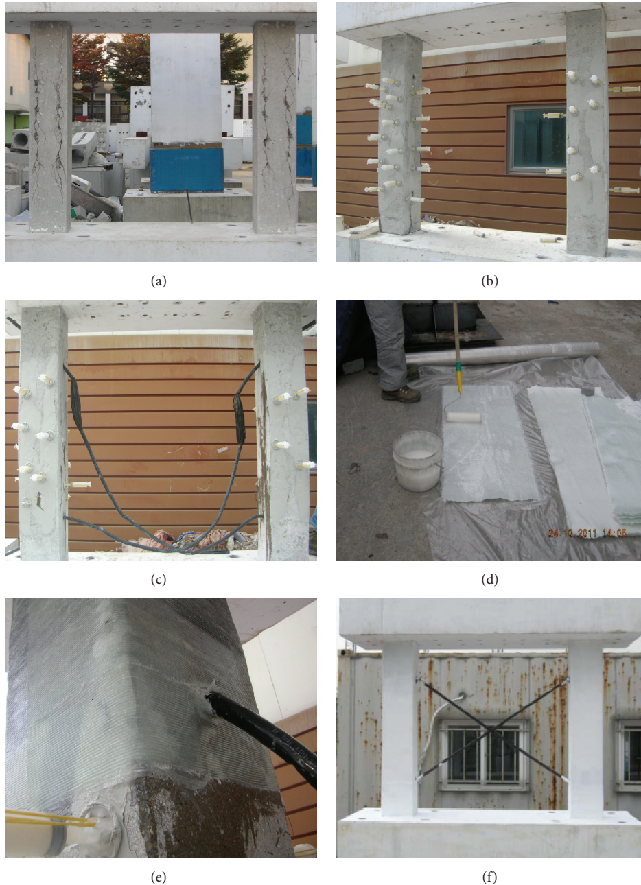
FIGURE 4: The fabrication procedure. (a) Control specimen with class-V damage, (b) surface treatment and injection of epoxy resin into the crack, (c) drilling of anchoring holes and installation of the CF X-bracing, (d) primer treatment process of the GF sheet, (e) externally bonded GF sheet wrapping, and (f) a specimen strengthened using the hybrid CF X-bracing and GF sheet wrapping system.
