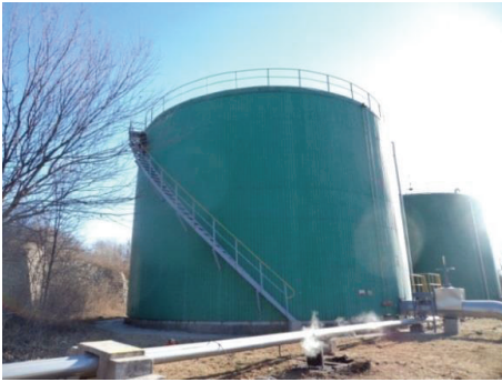
FIGURE 5: The fire-resistant water tank in field test.
