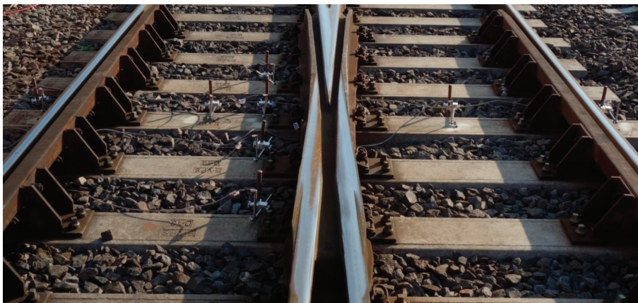
FIGURE 2: On-site installation of the sensors according to measurement methodology above.
